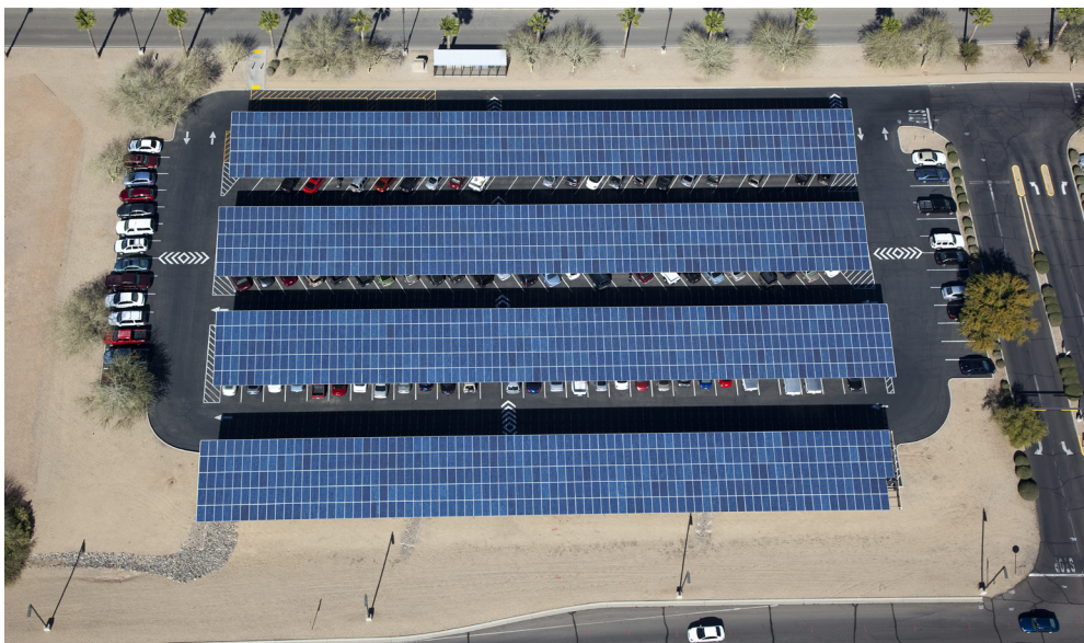
Figure 25 An example of solar covered parking, which provides the dual benefits of generating solar power while also shading vehicles
