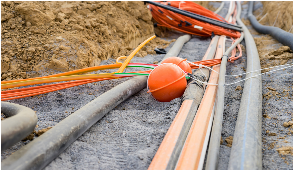
Figure 7 Wireline technology requires more disruptive installation processes, like that shown here, than wireless product options
